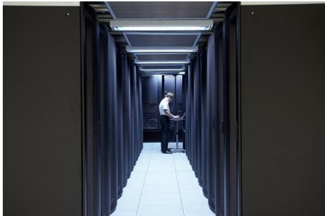
Contained Cold Aisle (AHF)
